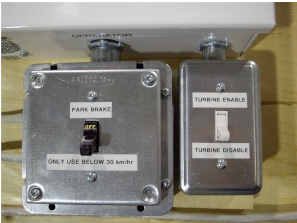
Figure 1: An example of a Raum 3.5kW wind turbine manual brake configuration.
